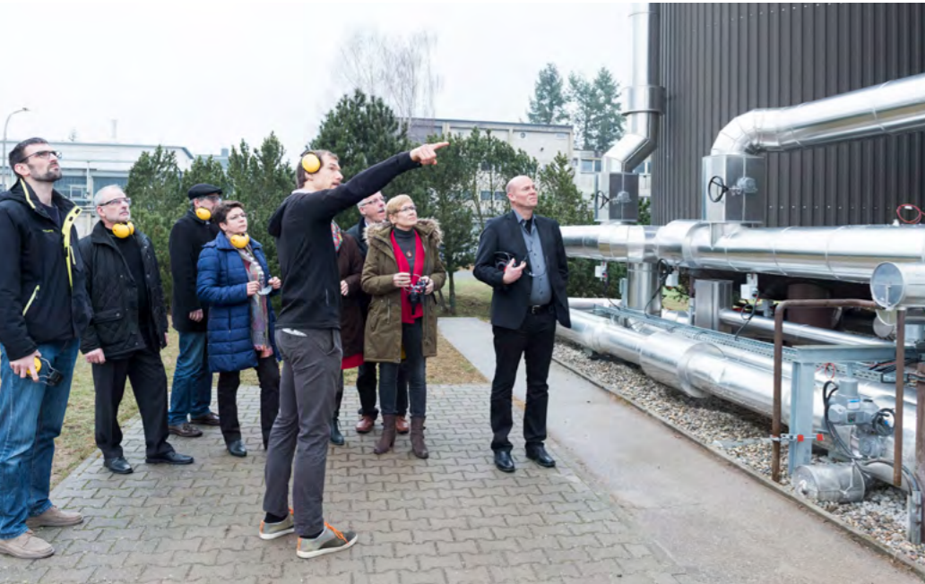
The new gas engine test laboratory and the cogeneration plant act as research platforms and sustainable infrastructure facilities on KIT Campus North.
